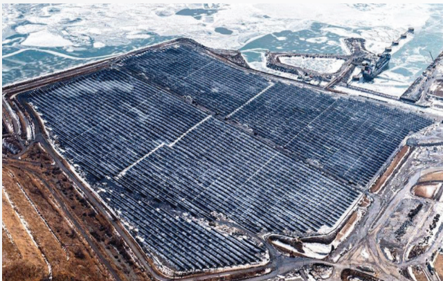
Solar PV plant at Nanticoke Generating Station, Canada
